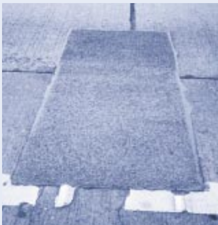
TechCrete installed after removal of the temporary repair. After two years it is still performing well.
